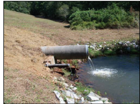
Forefront: toe drain pipe replaced this year
