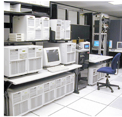
Network Operations Center
