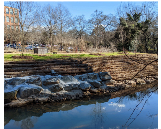
Figure 7. Brushy Creek after the implementation of boulder toe walls and soil lifts.
