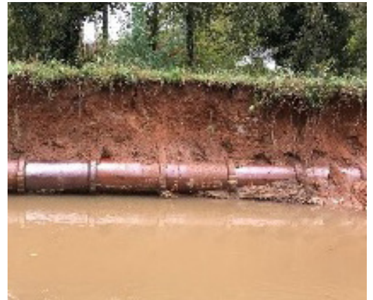
Figure 9. ReWa sewer pipeline exposed due to stream degradation.
